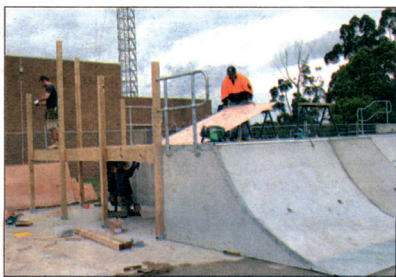
Ready to roll: Contractors installed new skatepark equipment in Churchill last month.
